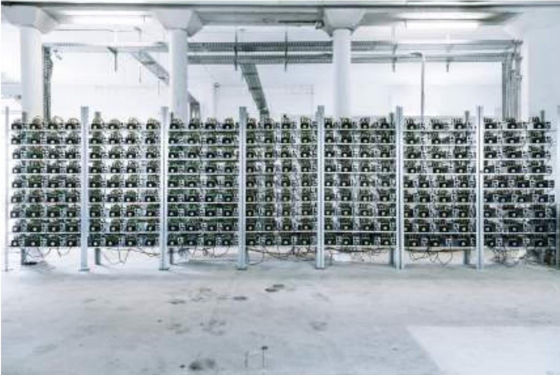
HydroMiner's facility near Waidhofen an der Ybbs, currently equipped with 250 ASIC miners (on view here) and 1152 GPU cards.
