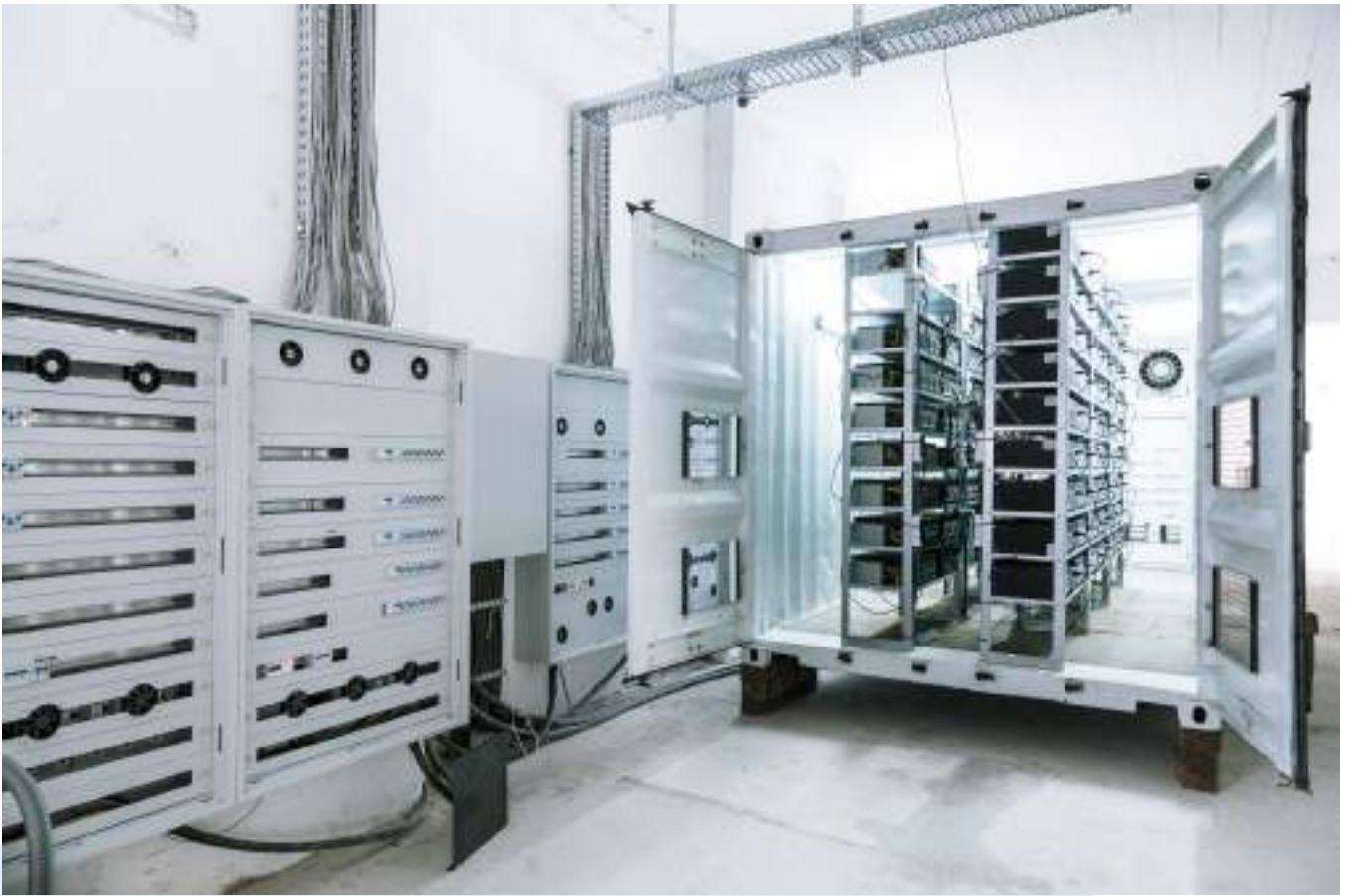
HydroMiner's container equipped with 1152 GPU cards and power connection distributing energy to the equipment inside the hydropower station.
